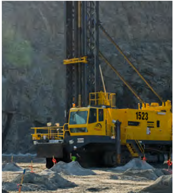
The typical hole spacing for the PV-351E is 7 x 9 m, drilling vertical holes to a depth of 19.5 m using two 9.9 m drill pipe in a single pass.
