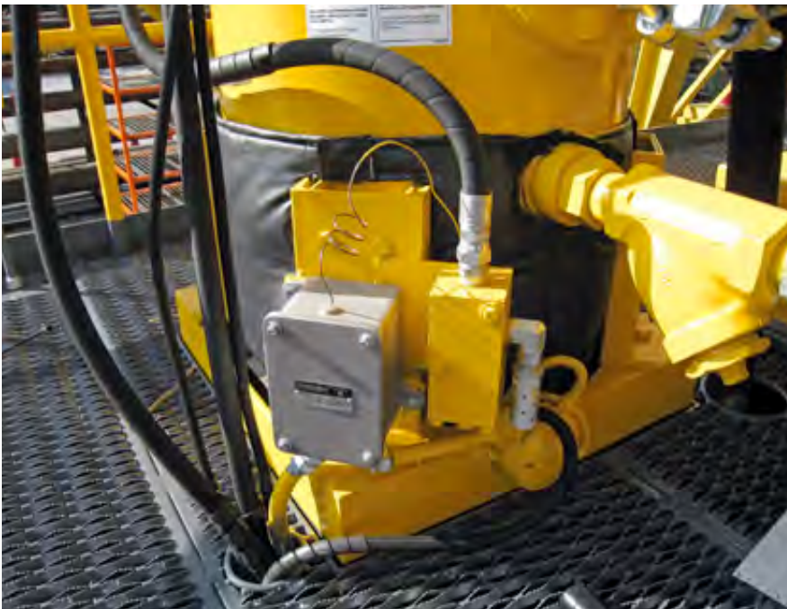
Cold package solution with heater blanket mounted on air receiver tank.
